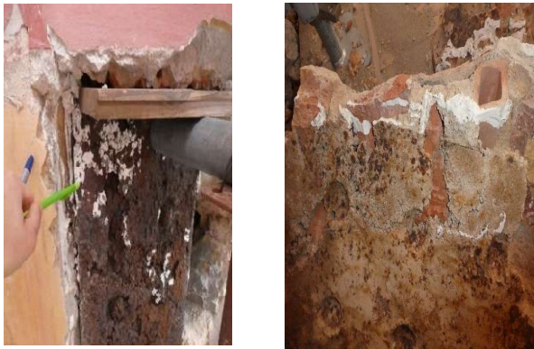
Fig. 2. a) Highly corroded surface, b) Materials, cement mortar and bricks with oxides
