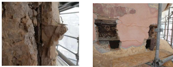
Fig. 3. a) Highly corroded surface of the steel column east side of the staircase, middle area, b) Corroded surface of the metal girder, near the roof east side
