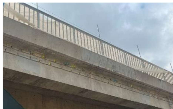
Fig.12. Installation of discrete drilled-in anodes on the downstream side beam of the deck
