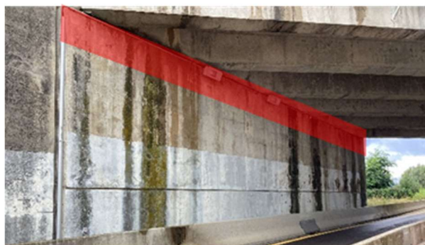
Fig.14. Treatment of the head beam on the abutment using discrete 600 mm drilled-in anodes
