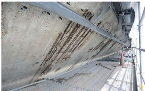
Fig.6. Sloping side veil of the front viaduct deck after preparation of the substrate by hydro demolition
