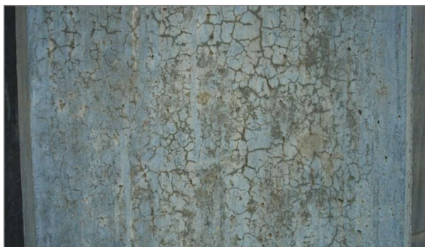
Fig. 1. Irregular cracking pattern caused by ISR.
