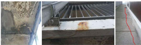
Fig. 10. Failing coating and joint + local rust stains + crack parallel to building (floor F16).
