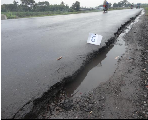
Fig. 1. Scouring occurs in a shoulder of rural road in Indonesia. A sign of "6" is a site number of a survey
