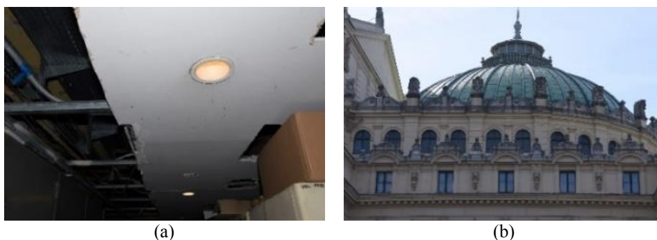
Fig. 6 a, b. Energy-intensive lighting and the Theatre's uninsulated roof (authors' own source).
