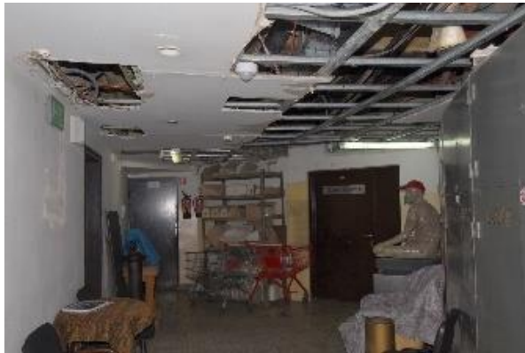
Fig. 4. The destroyed underground rooms of the Theatre, made in the 1980s (authors' own source).
