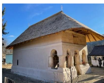
Fig. 23. The Holy Annunciation church at the end of the structural major interventions.
