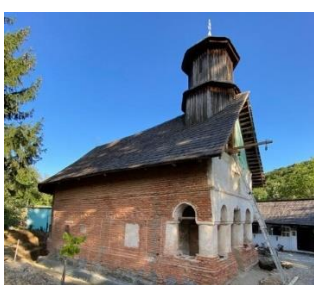
Fig. 22. Picture of the church at the end of consolidation of the foundations phase.
