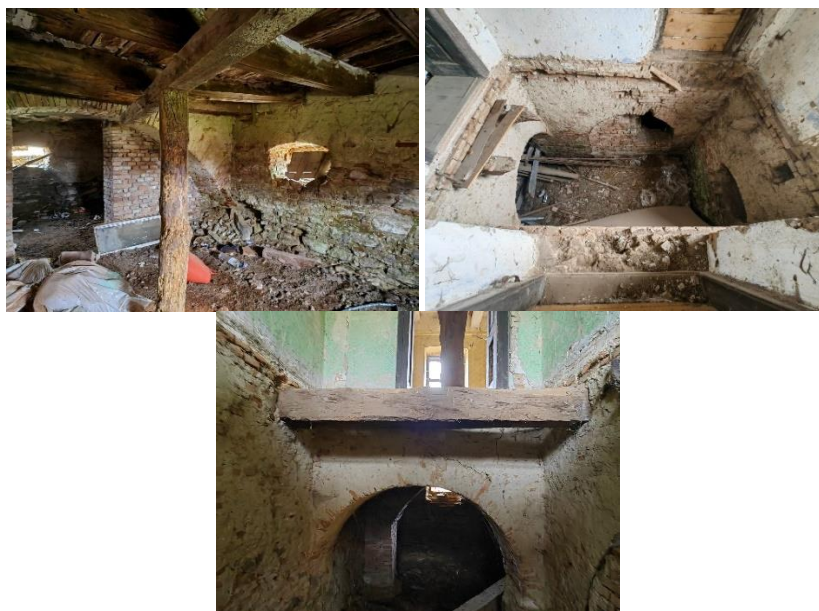
Fig. 11. Damage to the basement masonry arches and vaults.
