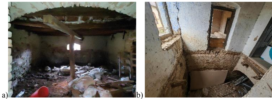
Fig. 13. Damage to the wooden elements: a) basement wooden beams; b) broken beam at the wooden floor.
