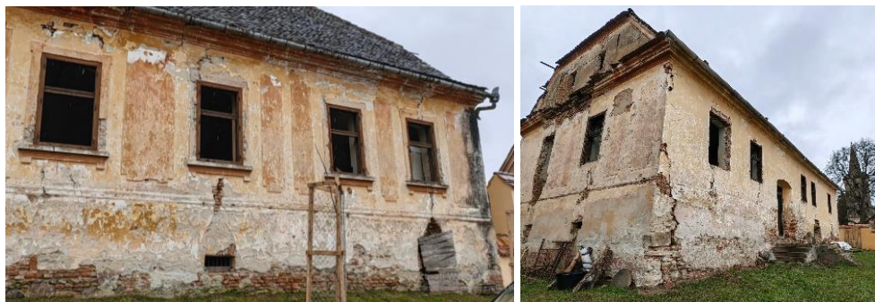
Fig. 10. Rainwater infiltration that led to the differential settlement of the foundations.
