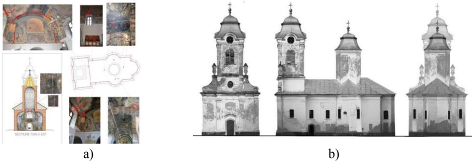
Fig. 2. (a) Cracks and degradation caused by differential settlements, (b) Deteriorations on the facades of Bezdin Monastery Church captured through 3D laser scanning
