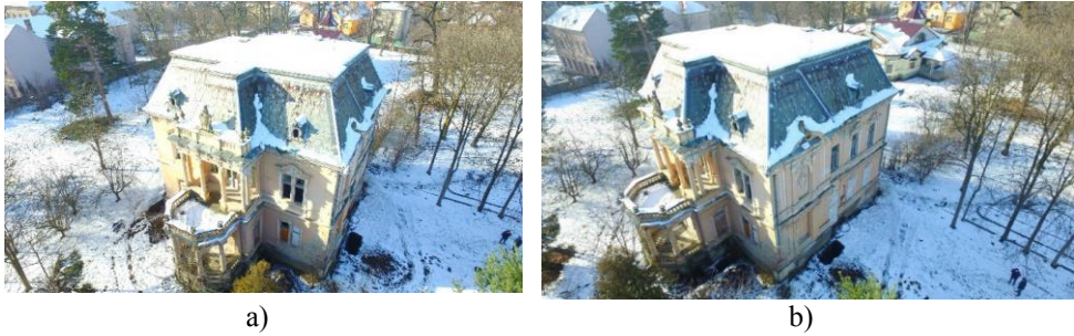
Fig. 9. (a) Cracks – South façade, (b) Cracks – North façade.
