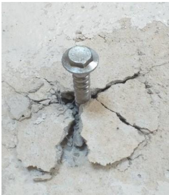
Fig. 12. Characteristic failure mode of the connection made observed in the tests screw anchors in the fibre reinforced concrete.
