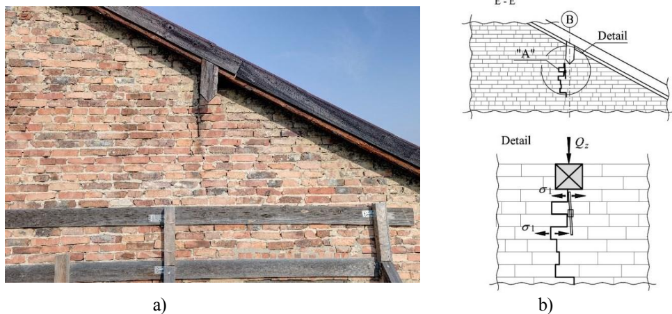
Fig. 10. Damage “E” to the wall in the axis 10: (a) photo of the damage as shown in Fig. 5, (b) the mechanism of damage occurrence.
