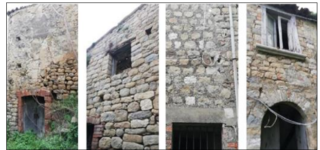
Fig. 4. Erosion phenomena on vertical masonry walls
