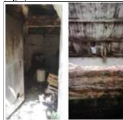
Fig. 5. Injured and deformed wooden beams
