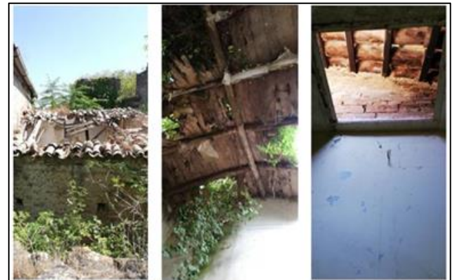
Fig. 6. Collapses of the roofs
