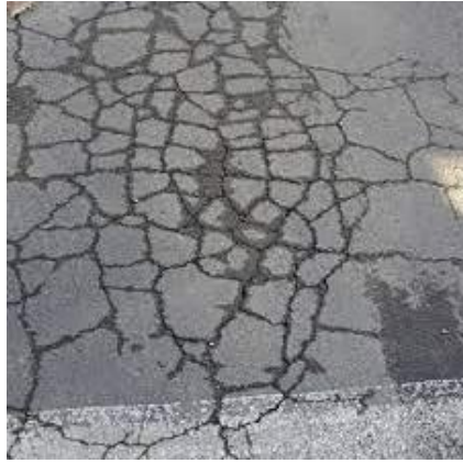
Fig. 1. Pavement deterioration due decreases in the subgrade's resilient modulus.
