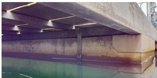
Fig. 9. TR-UHDC floating unit under the connecting frame of the pontoon, without any sign of degradation after 15 months of immersion in sea water in the Galway port area.
