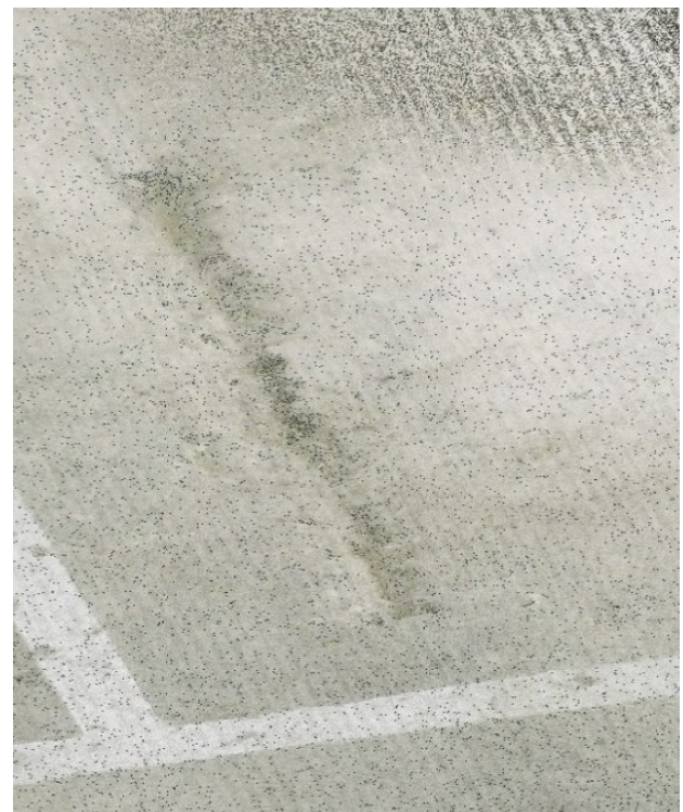
Fig. 6. Damaged area in point cloud
