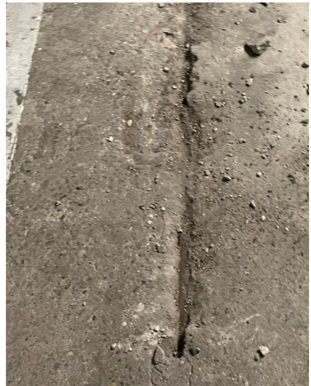
Fig. 5. Damaged area due to corrosion-induced spalling
