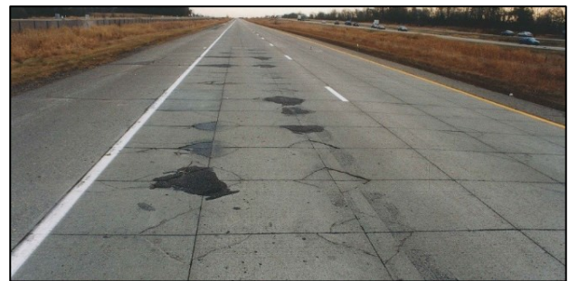
Fig. 4. Cracking on a COA-B overlay with longitudinal joints in the wheel path [11].
