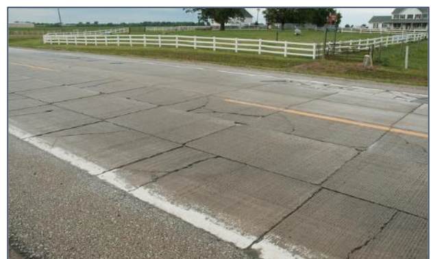
Fig. 11. Example of concrete overlay condition with 26.3% slabs cracked and significant fatigue damage [7].
