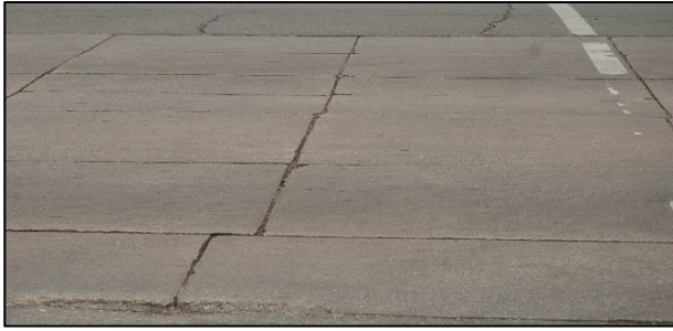
Fig. 6. Panel movement with transverse joints coming out of alignment with each other across several rows of panels [7].
