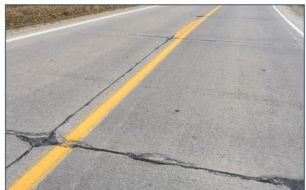
Fig. 2. Spalling of transverse joint and at joint intersections.
