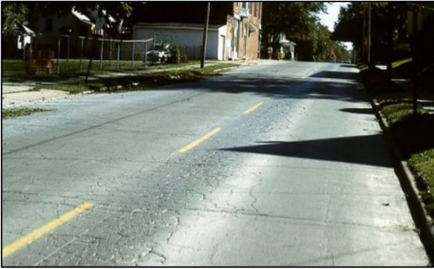
Fig. 8. Cracking after debonding of a COC-B overlay [10].
