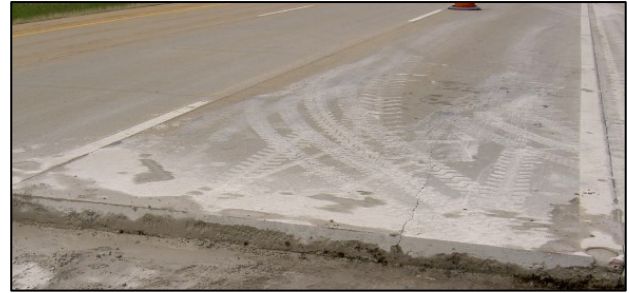
Fig. 9. Stripping of an asphalt interlayer (exposed in the foreground) leading to longitudinal cracking in COC-U [10].
