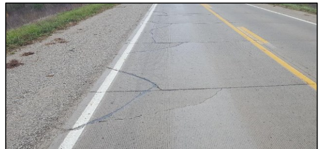
Fig. 3. Early age cracking on a COC-U overlay [5].
