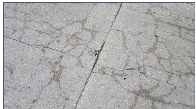
Fig. 1. Map-cracking at transverse joint.
