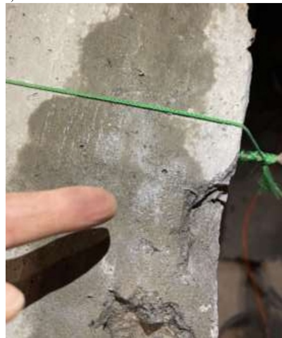
B) Along concrete crack above S7A1-S7B1
