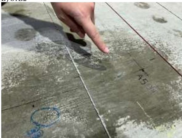
C) Along concrete crack above S1A1-S1B1
