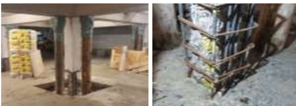
Fig. 1. extensive concrete replacement whilst the repair of a column in an underground car park according due to chloride-induced reinforcement corrosion
