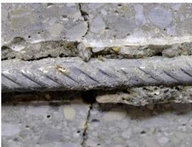
Fig. 8. 1.4003 Reinforcing steel in splitt concrete specimen with corrosion scar eccentric to separation crack
