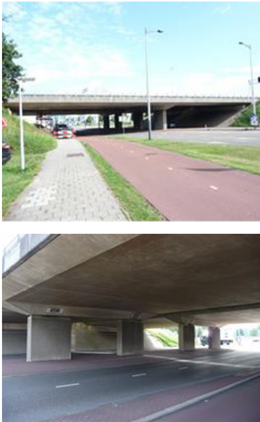
Fig. 2. Side view (top) of investigated bridge and columns supporting the decks (bottom)
