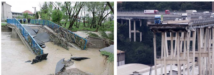
Fig. 1. Damaged bridges caused by a) extreme weather condition b) exceeding the service life
