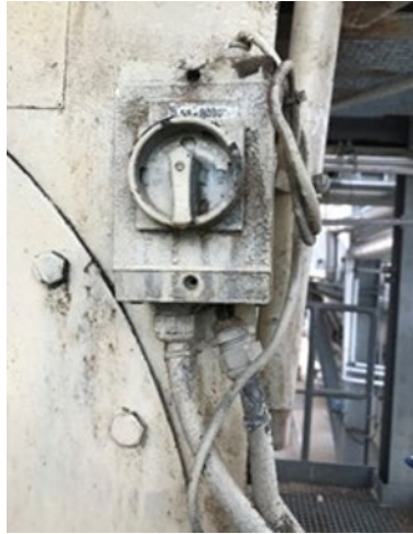
Fig. 5. Example of mandatory failure maintenance works.
