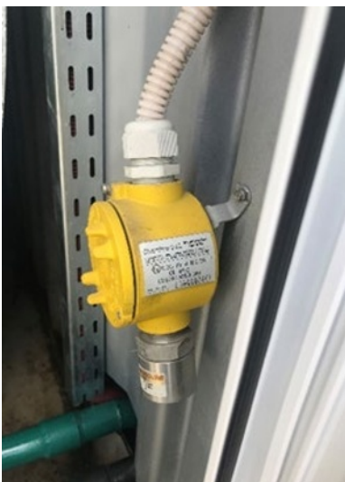
Fig. 3. Example of the improper choosing cable entry at the flame-proof equipment.
