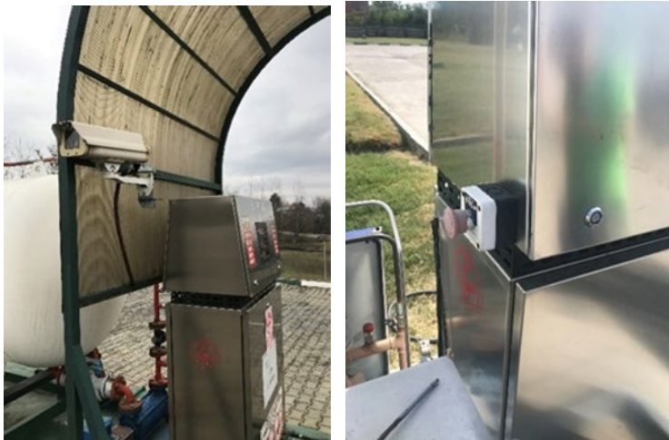
Fig. 1. Example of non-Ex equipment found in Ex classified areas, during site assessment visit.
