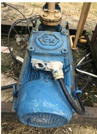
Fig. 4. Example of improper maintenance work applied to Ex equipment.
