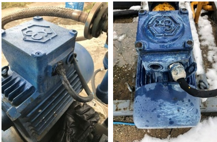
Fig. 2. Example of incorrect installation of electrical equipment in Ex construction.
