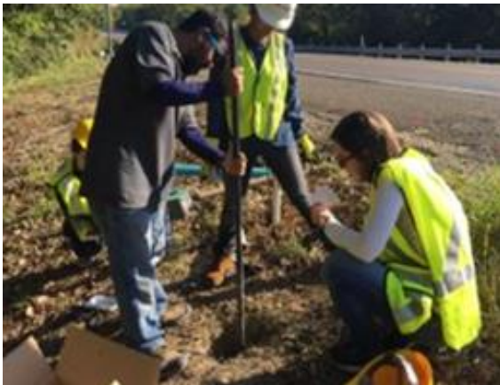
Fig. 3. Sensors installation at the study location
