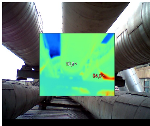
Fig. 3. The photograph and the thermal image of the piping system.
