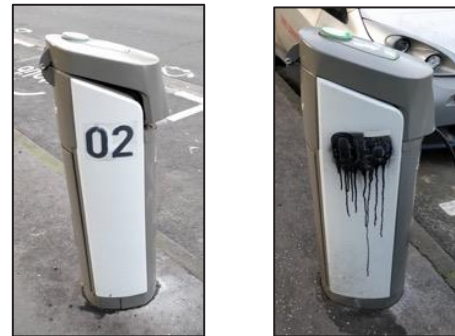
Fig. 3. Two plug-in platforms that has been subject to vandalism in France
