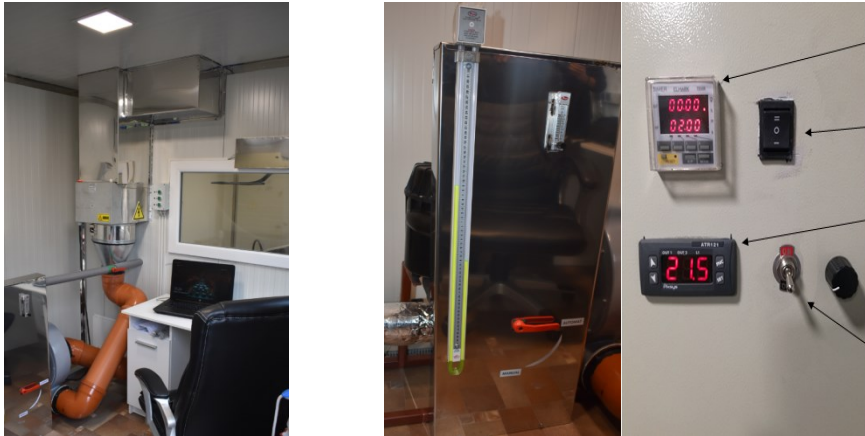
Fig. 3. Command room with Flow Control / Pressure / Control Panel
