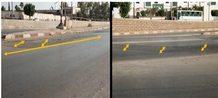
Figure 1: Important deformations of a section of RN4 express road in Chlef city (Algeria)
