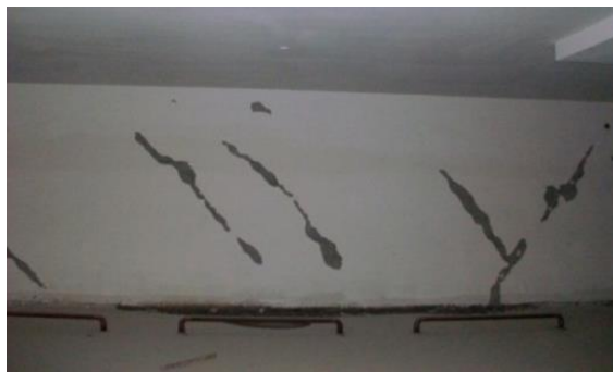
Figure 3. Cracks on a concrete shear wall
