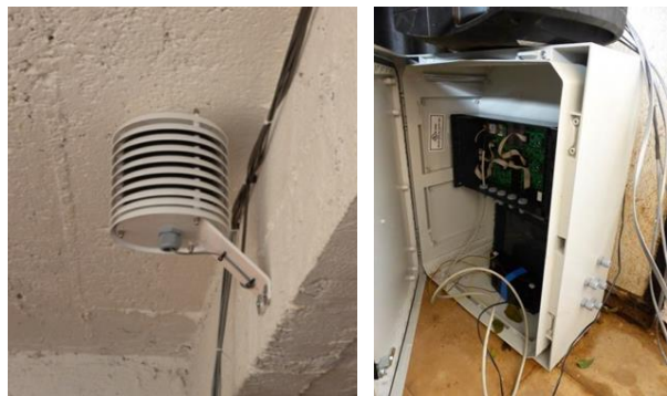
Fig. 4. Weather station (left) and data acquisition system remotely accessible (right).
