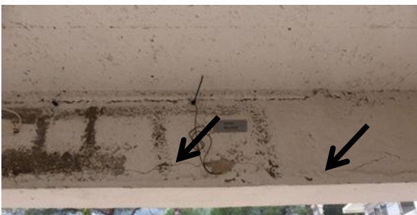
Fig. 16. Opening of a crack on the beam in the vicinity of the measurement point B23.
