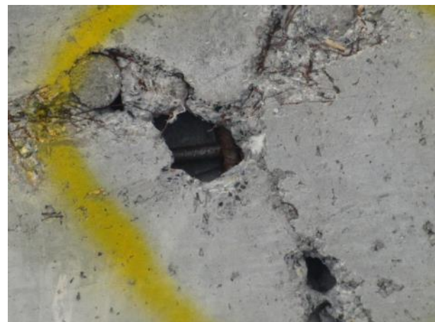
Fig. 3. Honeycombing with visible reinforcement
