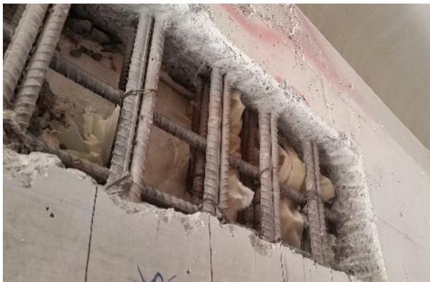
Fig.10. Debris below void former
