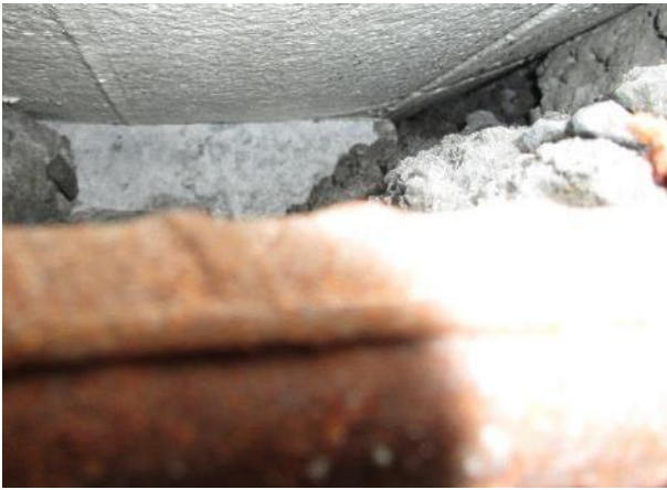
Fig.4. Void below void former and non-embedded rebar
