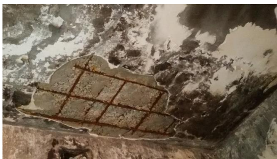
Fig. 2. Exposed rebars and delamination at Room-9 of Fig. 1.
