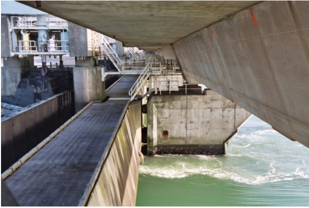
Fig. 1. View of the location and exposure conditions of the walls of the box girder bridge.
