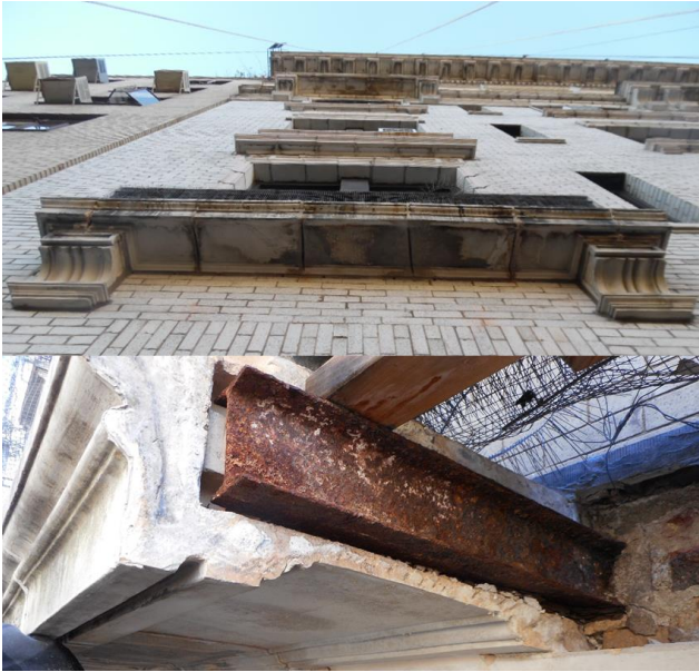
Fig. 2. (Top) Terra Cotta Balconettes. Fig. 3. (Bottom) Exposed Corroding Outrigger.
