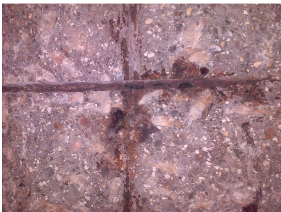
Fig. 5. Chloride pitting on the steel broken out during the repair of H6 canal bridge
