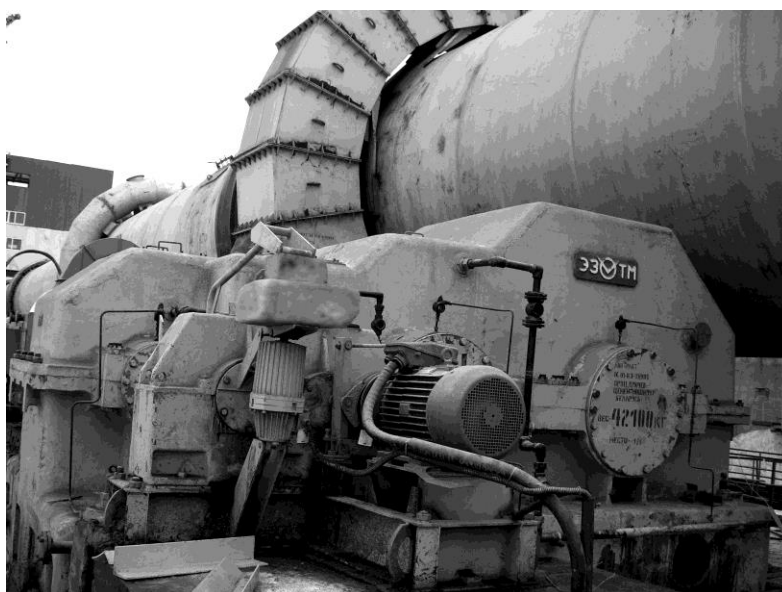
Fig 1. Drive of rotary kiln Ø4.5x170m with reducer CT-3230.
