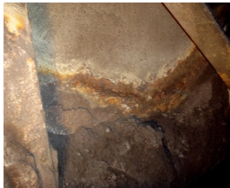
Fig. 8. Strong pitting corrosion of the steel sheet.
