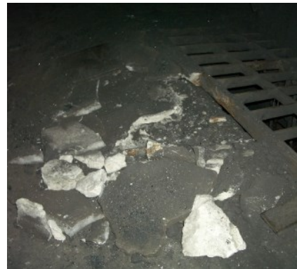
Fig. 14. Strong mechanical damage of the concrete floor.
