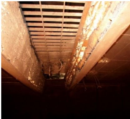
Fig. 13. Corrosion and mechanical damage of the beams supported cover plate.
