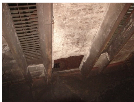
Fig. 3. Steel beams (with a concrete cover) serving as a support of the upper slab.
