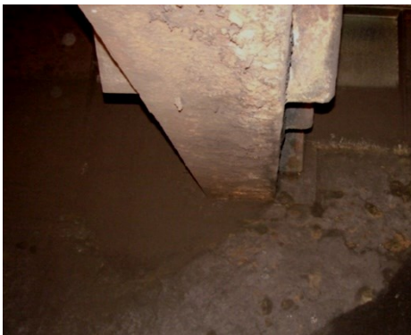
Fig. 7. Surface corrosion of the plain girder.
