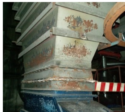
Fig. 12. Mechanical damage of the hopper's external surface.
