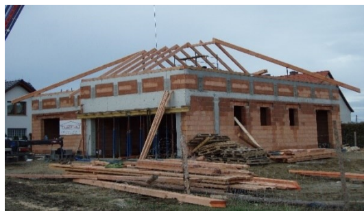
Fig. 9. An example of a residential building with improved stiffness, i.e. with two concrete rim and selected concrete columns.
