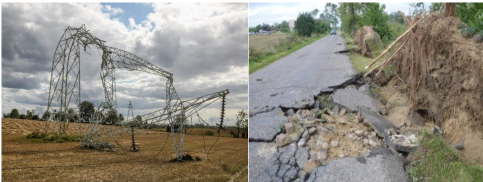
Fig. 7. Damage to a overhead power line pole and a commune road.
