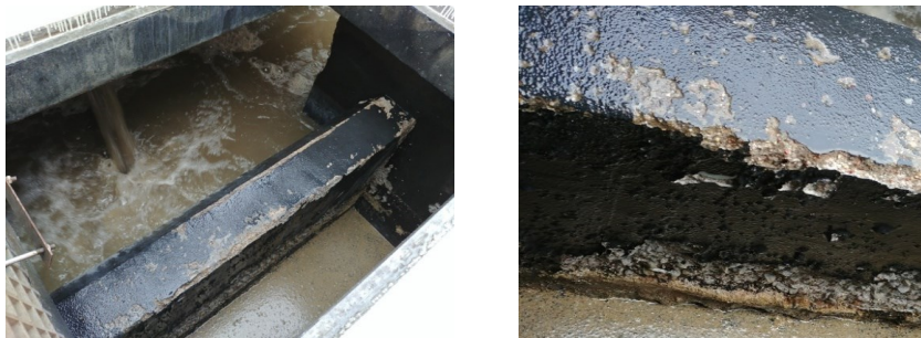
Fig. 5. Damaged surfaces of walls of the tank 01/1.
