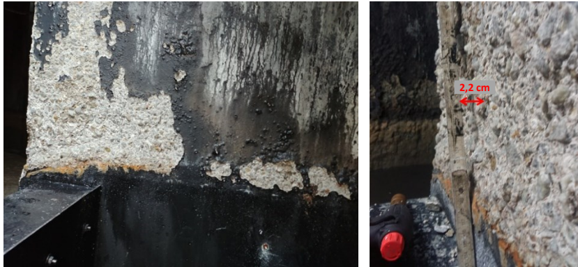
Fig. 7. Damaged surfaces of walls in tank 02/2.
