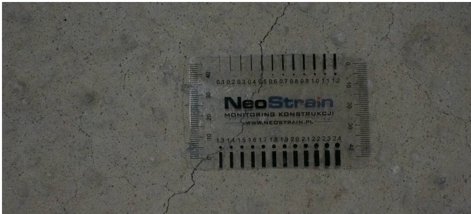
Fig. 10. Measurement of the cracks in sample no. 4.
