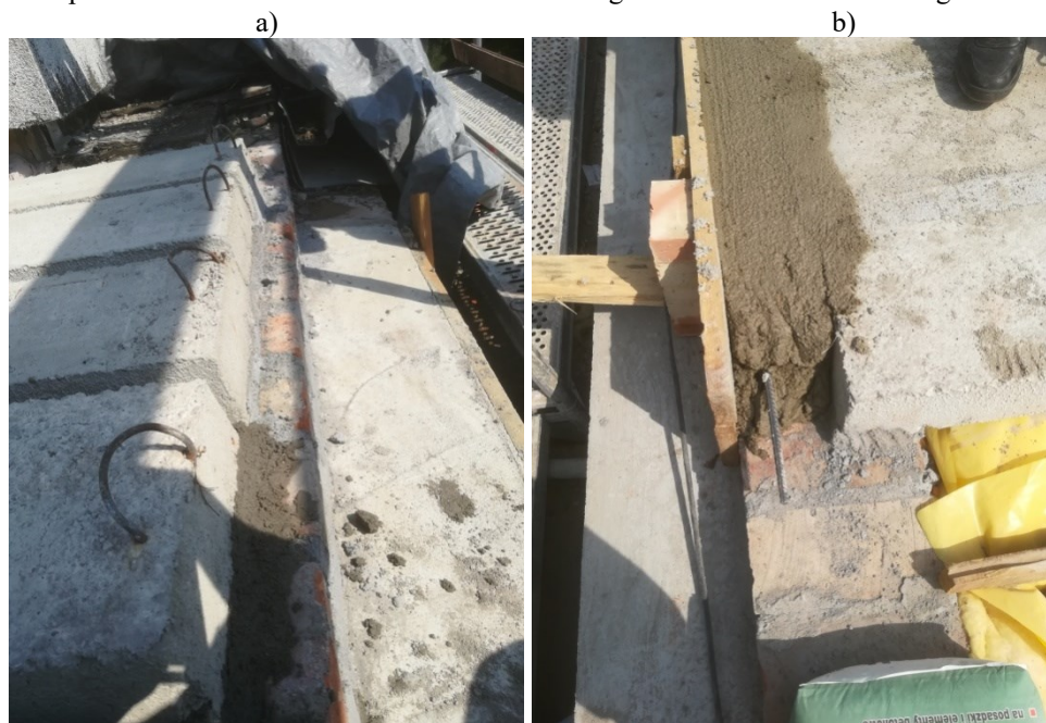
Fig. 11. The structure of the roof a) channel roof slabs, b) the ring beam around the slabs.
