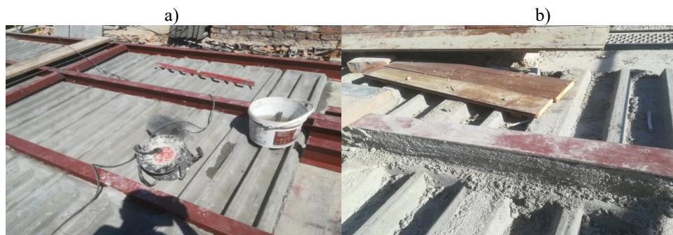
Fig. 10. Reconstructed structure of the ceiling over the last floor a) WPS slabs laid on steel beams, b) fillet welding of slabs.
