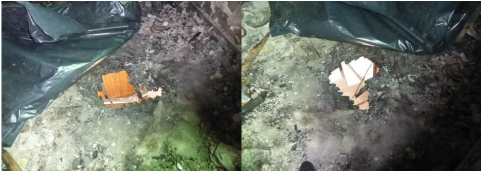
Fig. 8. The damage of the ceiling slab between apartments no. 106 and 109.
