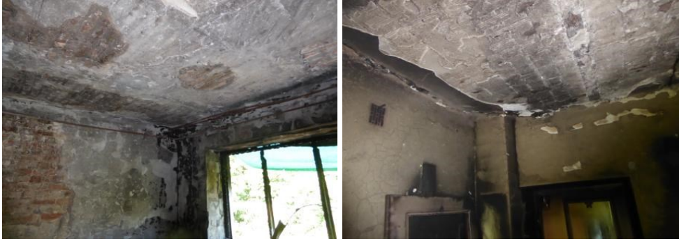
Fig. 7. The interior of the apartment no. 109 after the gas explosion.
