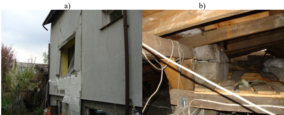
Fig. 2. Building elements, that acted as explosion relief openings while gas explosion a) window in the kitchen room, b) roof structure.
