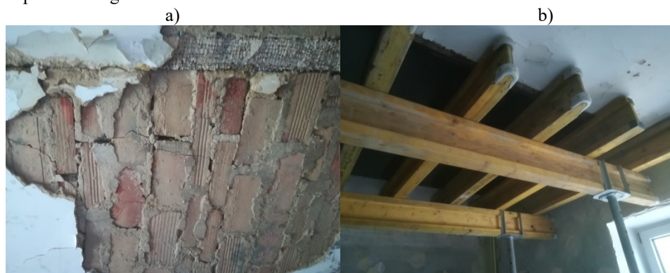
Fig. 12. The ceiling above the kitchen room in the apartment no. 106 a) the broken ceiling slab, b) formwork under the reinforced concrete slab.
