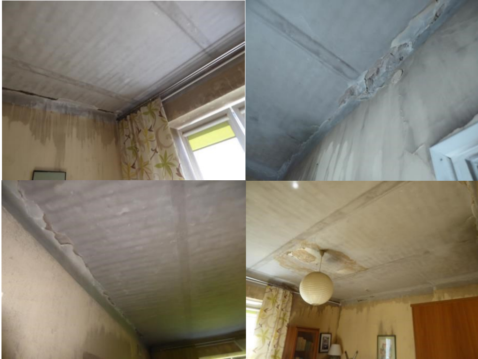
Fig. 5. Examples of damage of joints between walls and ceilings in the housing unit above the last floor.
