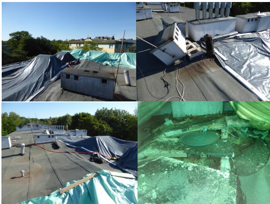
Fig. 4. The condition of the roof structure of the building after the explosion.
