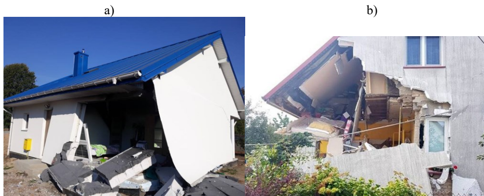
Fig. 3. The condition of single- family houses after the non-vented gas explosion a) residential building in Orzechowice [6], b) residential building in Hajnówka [7].
