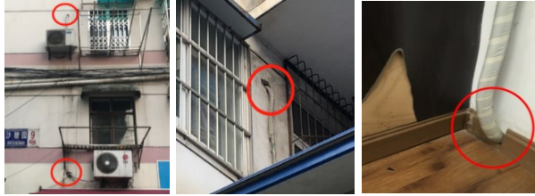
Fig. 1. Air cavities due to air conditioners of the buildings in Nanjing
