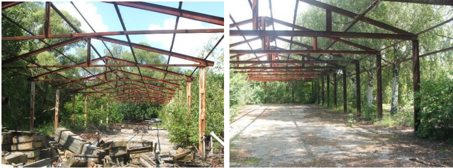
Fig. 1. Corroded steel structures which elements may using again.
