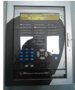
Fig. 3. New digital relay protection for generator.
