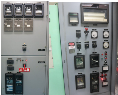
Fig. 2. Electromechanical relay for generator protection.
