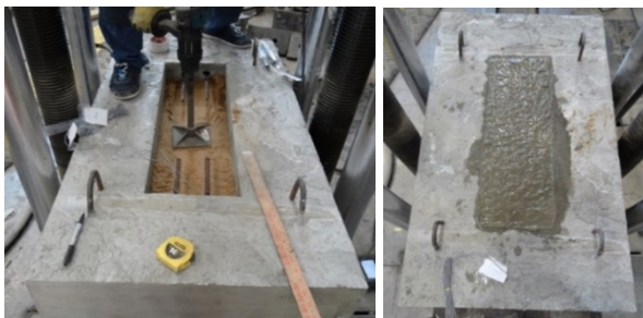
Fig. 5. (left) Placing and compacting of sand and (right) cast-in-place PC punch test specimen.
