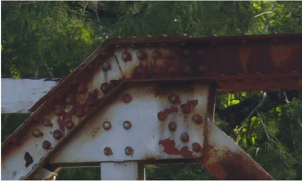
Fig. 4. UAV view bridge corrosion.
