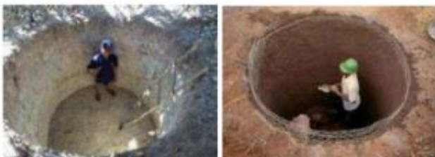
Fig. 9. The rainwater tank made from ferro-cement.
