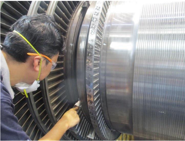
Fig. 8. Reblading of welded slots. The weld repaired and machined seal area can also be seen in the photo on the right.
