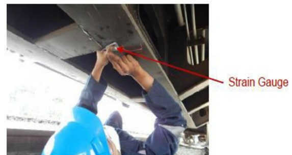
Fig. 17. Assembly of strain gauge on the underframe wagon based on FEM analysis.
