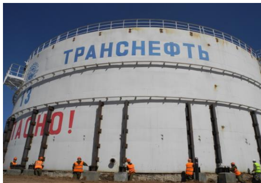
Fig. 2. A reinforcing frame of a special configuration for lifting the vertical steel oil storage tank.
