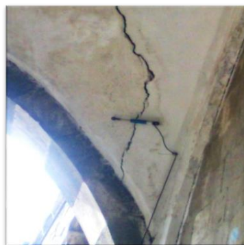
Fig. 2. Cracks in the cupolas of Suleiman Tikie.
